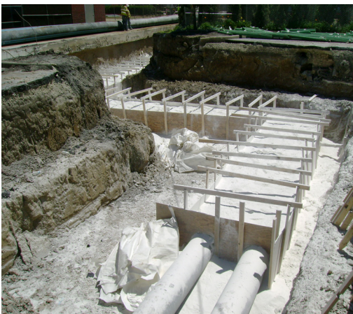
Typical DriTherm application prior to backfill. (Forms are not required except to minimize material usage.)
